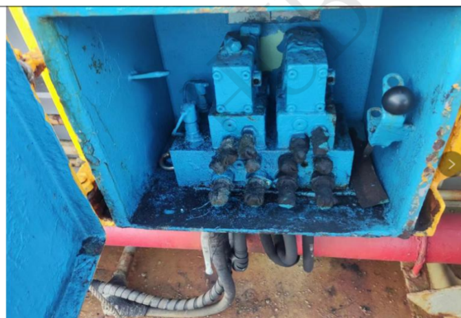
the condition of the control valve block
