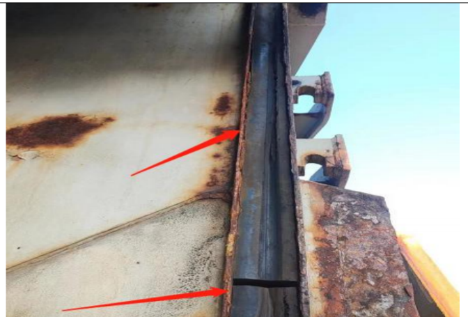
the condition of rubber packing
