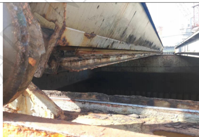
Rubber channel was rusty
