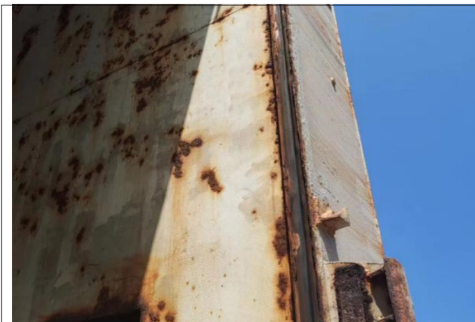
the condition of the HC backside and skirt plate
