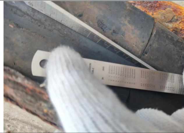
the condition of rubber packing
