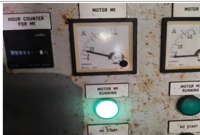
Electric current of the pump
