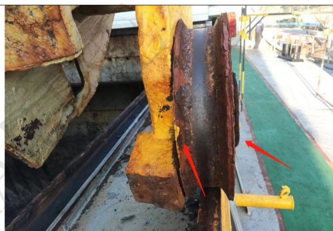
Running wheel was worn out heavily
