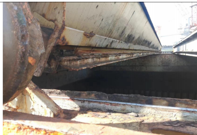
Rubber channel was rusty
