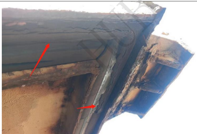
the condition of rubber packing
