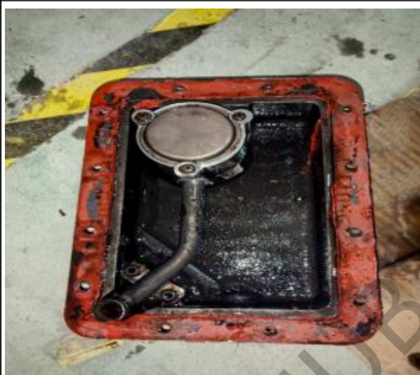
The No.1 oil pan has too much waste oil.
